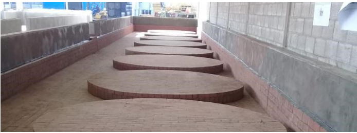
4. Finished sulfuric acid storage tank farm secondary containment area protected against corrosion with acid-resistant brick, FURALAC Green Panel Mortar, and TUFCEM II SL Membrane.
