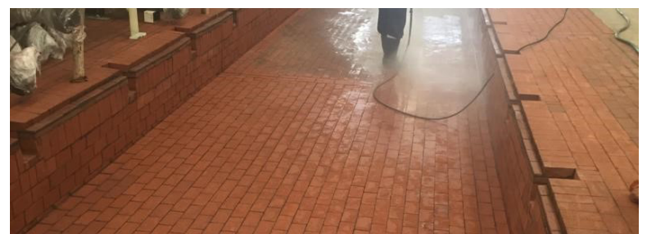
2. Finished battery filling area trench lined with acid-resistant brick, FURALAC Green Panel Mortar, and TUFCEM II SL Membrane.
